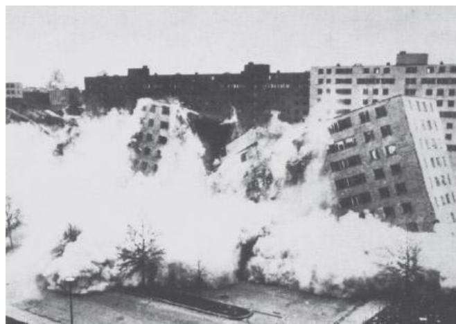
Partial demolition of Pruitt-Igoe housing complex (Leinweber, Yamasaki & Hellmuth, 1950–54), St. Louis, Missouri, 1972.
